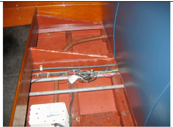
Wiring bundle and routing
